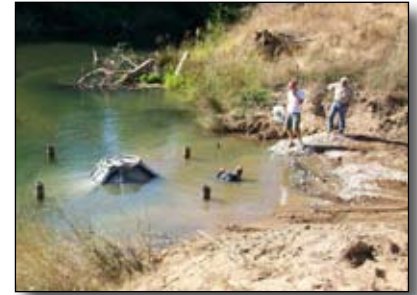
Fish Screen at the North Pumping Station
