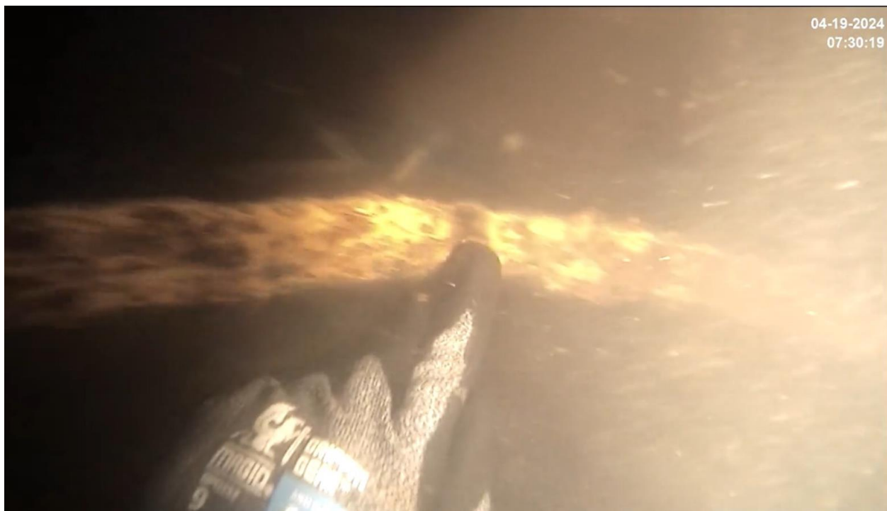
Solid Seam in the Tracy Lake 48 inch CMP supply line
