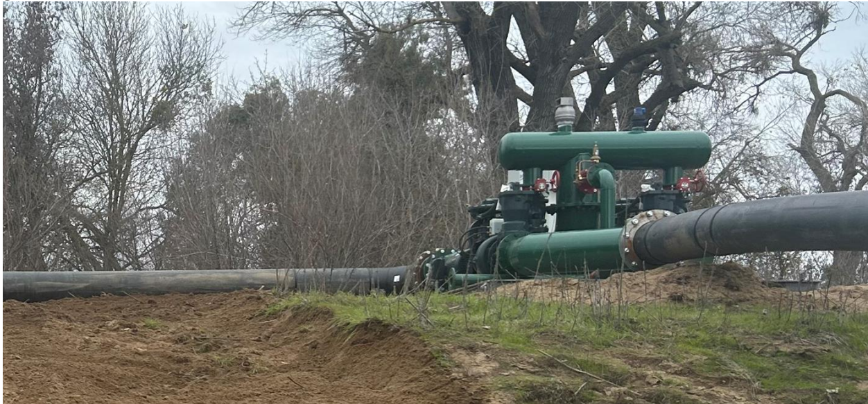
New North System Temporary Pump Station
